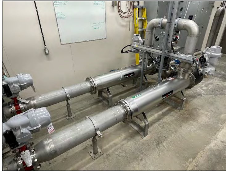
Panorama UV disinfection units
