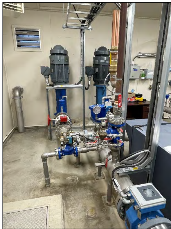
Treatment Station Booster Pumps
