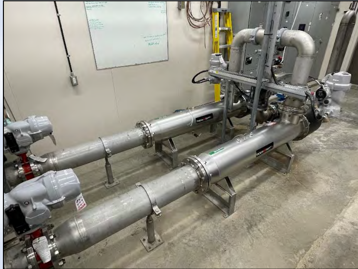
Panorama UV disinfection units
