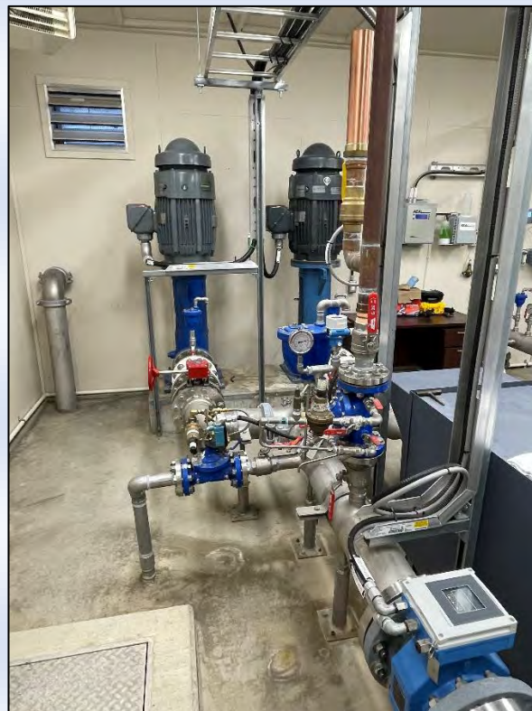
Treatment Station Booster Pumps
